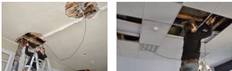
Fig. 2 Evaluation of the bottom chords of the trusses of roof with the Microsecond timer
