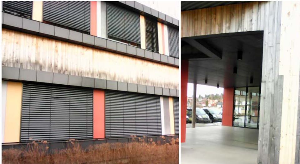
Figure 8. School in Ås as example of weathered structure
