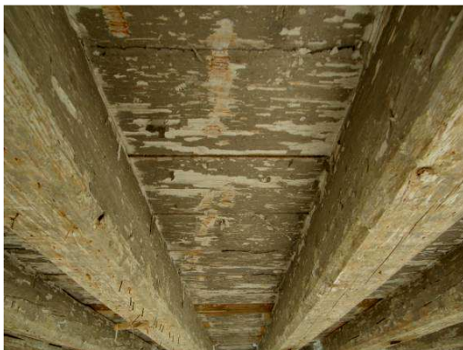
Fig. 4 Remnants of the original surface of ceiling beams after removal of the falls ceiling
