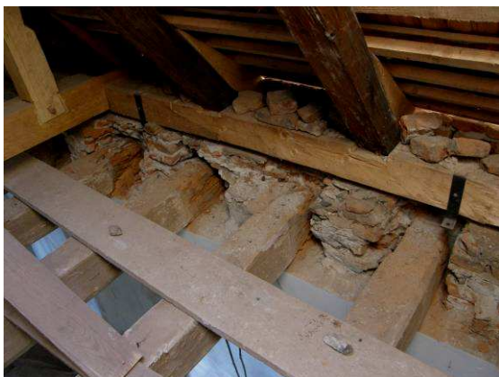
Fig. 6 The beam heads damaged by brown rot fungus
