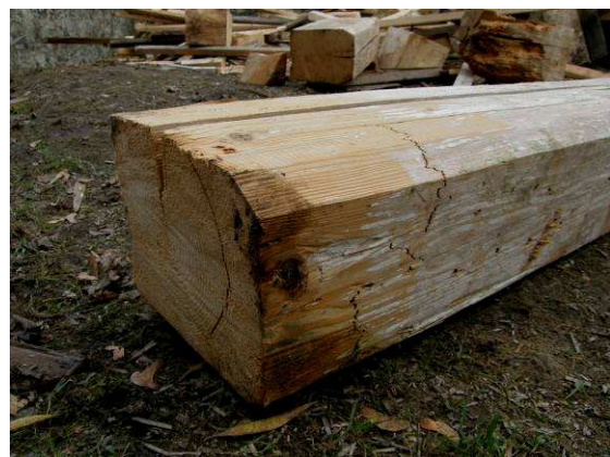
Fig. 7 Detail of the transversal crack in the lower part of beam
